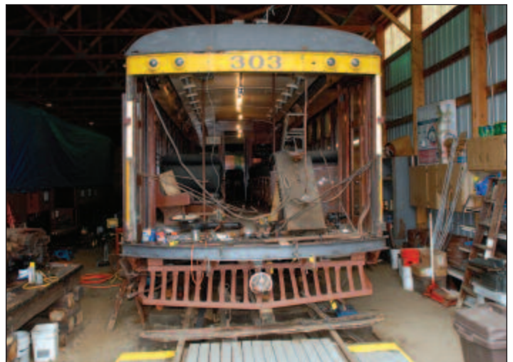
▲ In NORM's barn the smashed front end has been removed from car 303 and new steel has been fitted into place on the frame and front bumper. —NORM Collection
